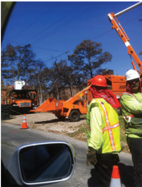
Tree trimmers cut branches away from power lines in an effort to prevent more wildfires in the Bastrop, Texas, area.
